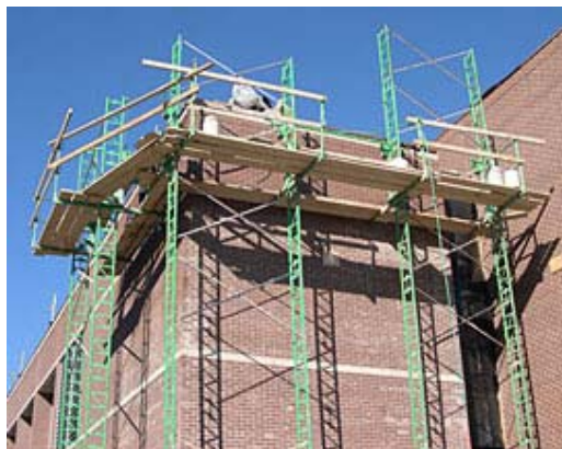
McKinney Masonry uses Non-Stop Junior scaffolding as a way to work faster and double profits.
